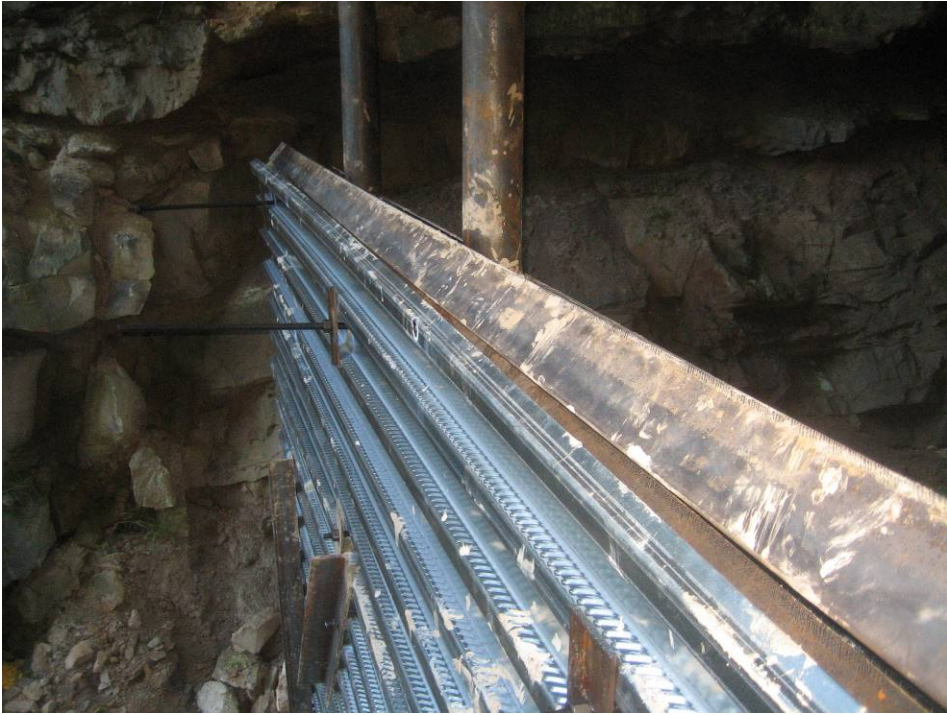
Figure 3. Air barrier partially built with vertical supports, bat gate, and start of welded steel exterior.
